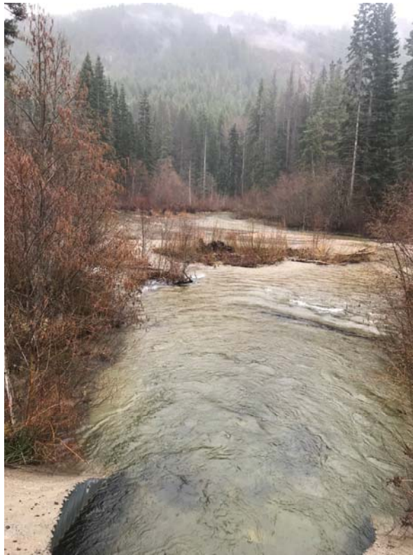
Figure 15. Sedimentation at outlet of upstream culvert to historic channel (photo from April 2018).
