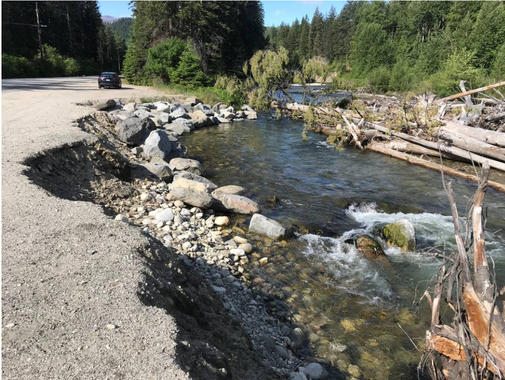
Figure 10. Area 2 in June of 2018. Note erosion behind rock revetment, and tree that was upstream in April now at logjam.
