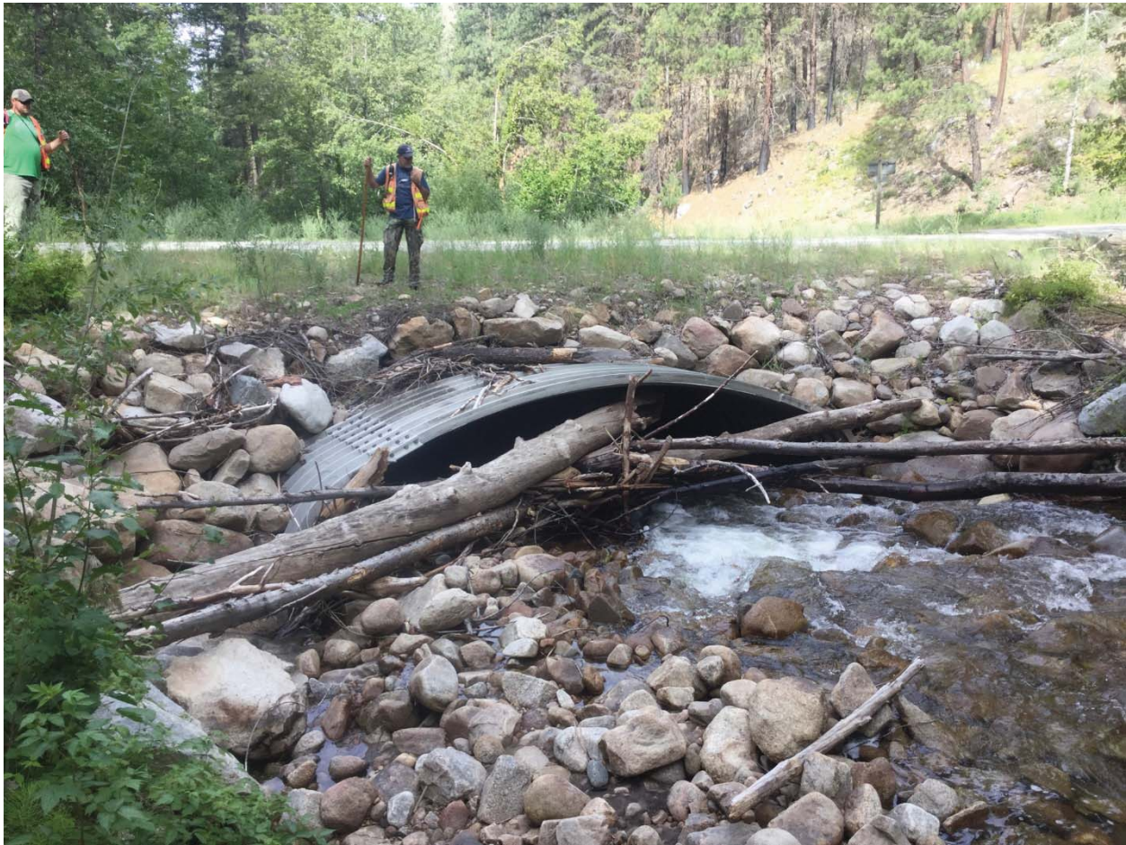
Figure 2-6. Photograph of Wood Racking at Culvert Crossing Inlet on NF-4225 Road near RM 9.5
