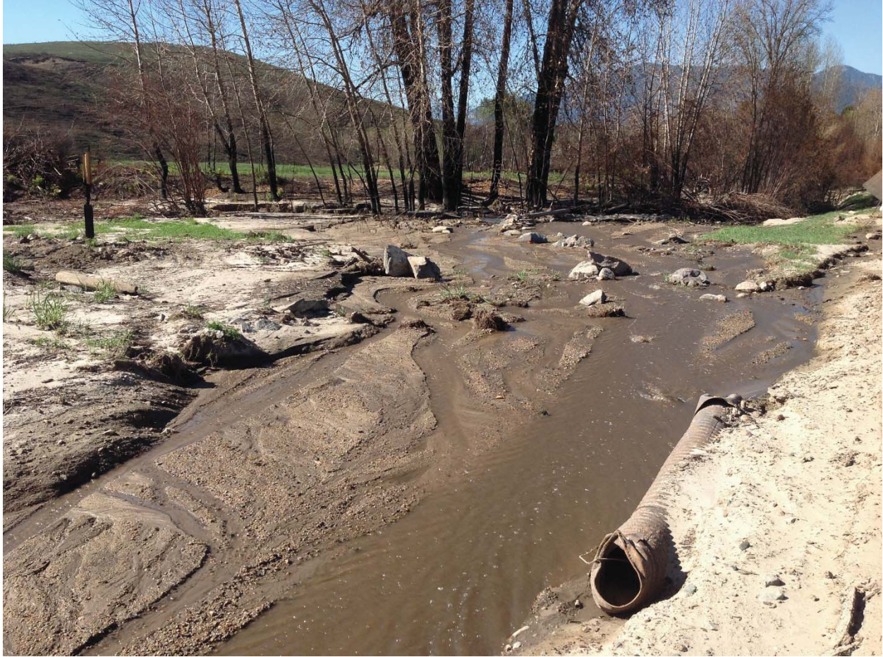
Figure 2-9. Photograph of Road Drainage Failures and Surface Erosion at Storer Creek (Reach 4) Following the Carlton Complex Fire (Source: BAER 2014)
