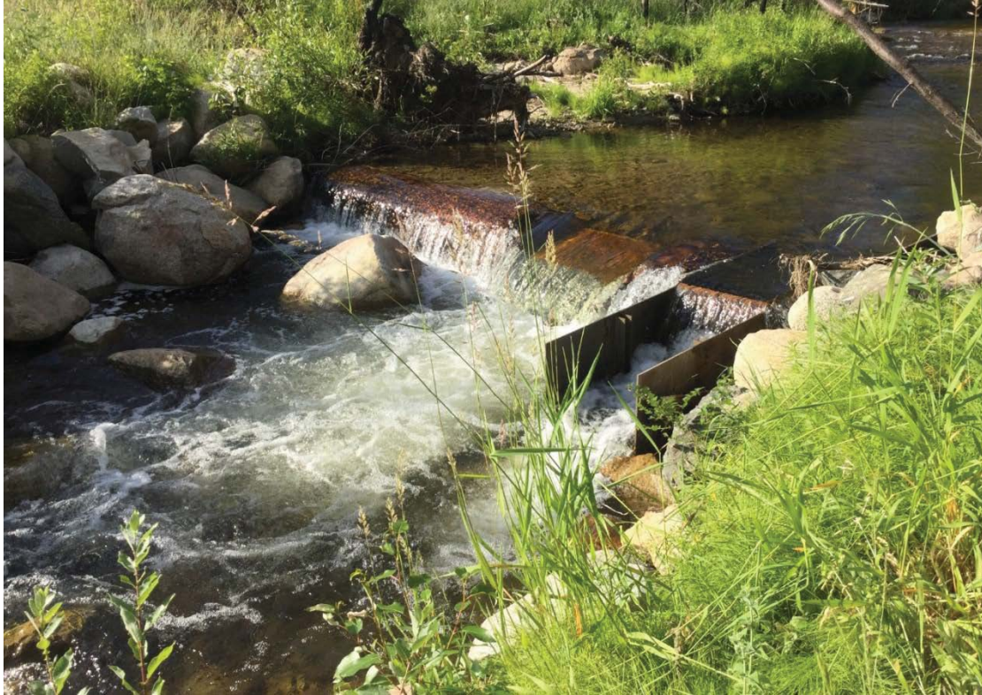
Figure 2-3. Photograph of Log Weir and Ladder Structure near RM 6.3 at Batie Diversion
