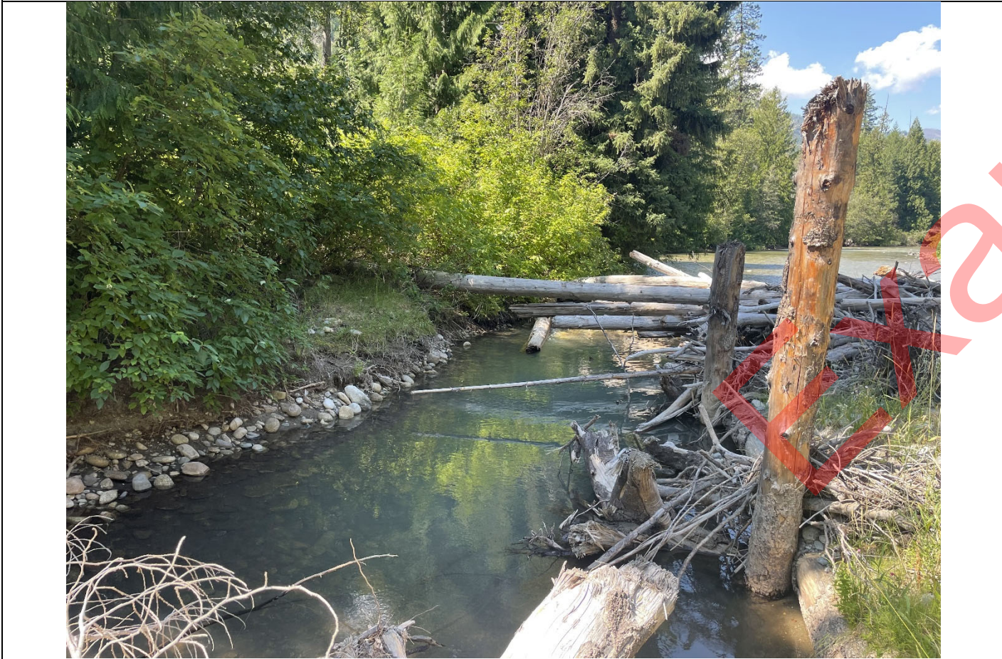
Significant large woody debris accumulation at face of inlet structure formed in 2023. The obstruction is still not limiting fish passage as there is a deep pool under the wood and the corner of the LWS, which is intact. See next photo point for additional comments.
