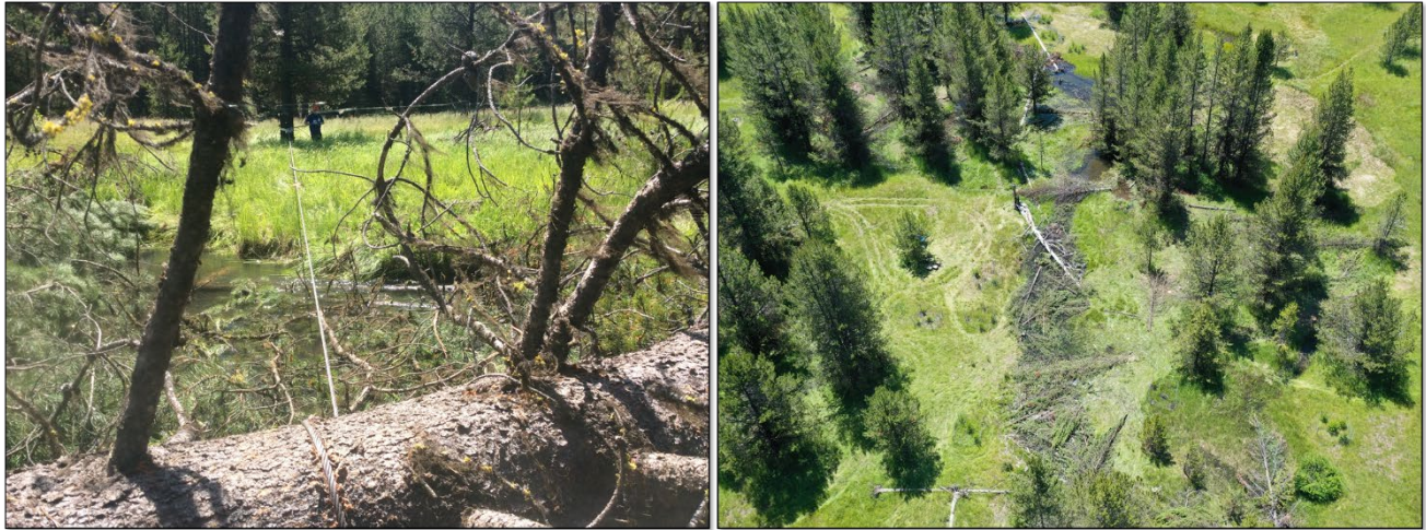
Figure 12. Utilizing a griphoist to move large wood from the adjacent floodplain into the stream channel (left photo) and example of high densities of large wood left unanchored in the channel and placed on the floodplain to add roughness (right photo). Photo examples are from restoration on a tributary to the upper Grande Ronde River in Oregon.
